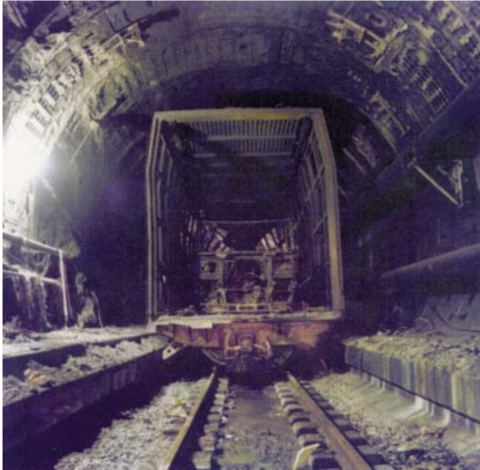
Figure 1. Aftermath of the Channel Tunnel fire in November 1996 (Photo courtesy of Eurotunnel/QA Photos Ltd).
